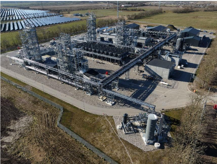
European Energy's Power-to-Methanol plant in Kasso, Denmark. © European Energy
